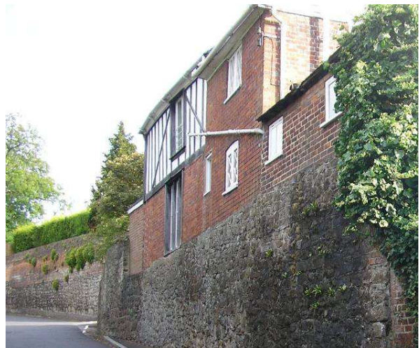
Soil pipe on Bank House
